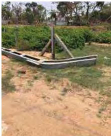
Figure 6.2: Damaged Steel H-Pole
