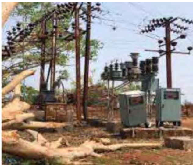
Figure 6.1: Damaged 33 kV Panel and Substation
