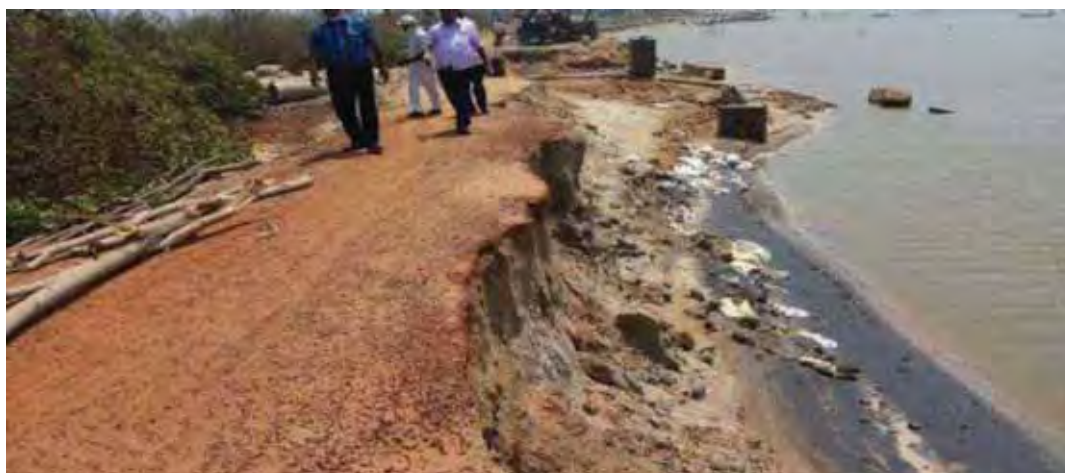
Location: Brahmagiri Block, Puri District – damaged section of Nadiakhai Saline Embankment
