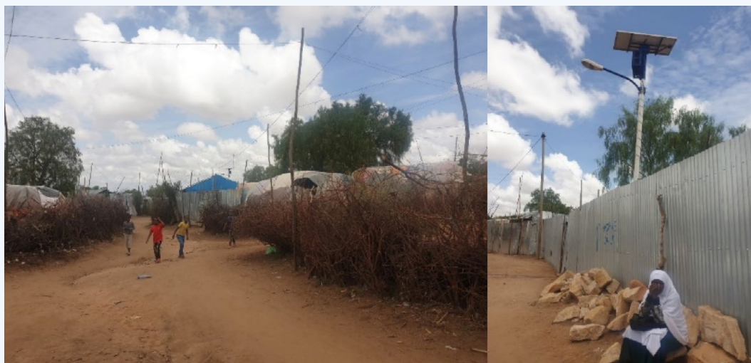
► Photo 3. Solar panels and informal grid connections in Kebribeyah
