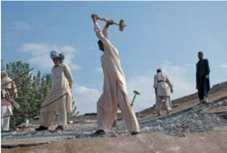
The town of Mansehra, 50 km north of Islamabad, was badly affected by the earthquake. Demolition and recovery is underway to salvage as much material as possible for new construction.
