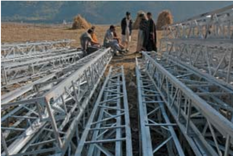
Rebuilding electrical networks in Balakot. New steel towers were delivered quickly to help restore communications.
