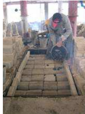
Figure 19. Fireman adding coal to unfired bricks This process is unique to eco-kiln.
