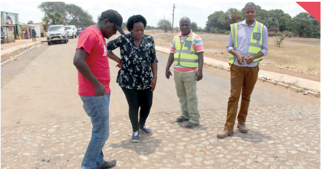
ILO consultant Caroline Naliaka-Maina, ILO Programme Assistant Hastings Chijikwa and Zambia Sugar project engineers check on the portion of the road done with cobalstone by the community.
