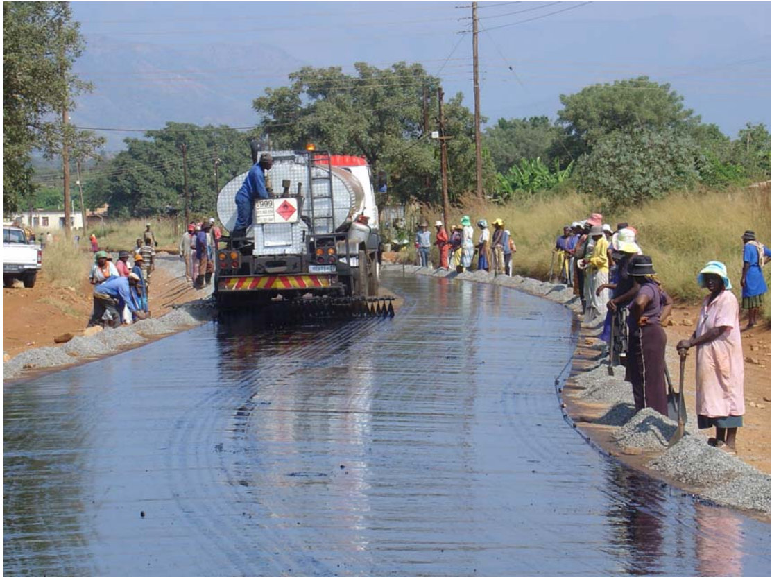
Figure 4: Spraying hot bitumen for Otta- or Grav Seal. Aggregates are spotted along the road and labourers waiting to spread.
