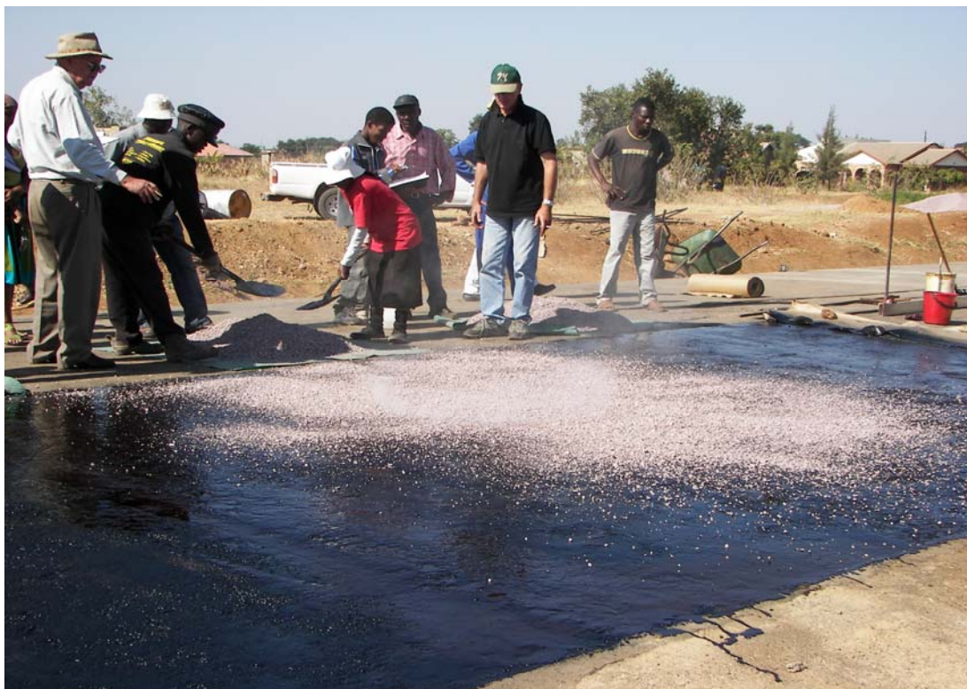
Figure 8: Manual spreading of aggregate requires a good technique and careful brooming and backchipping to ensure the entire area is covered uniformly
